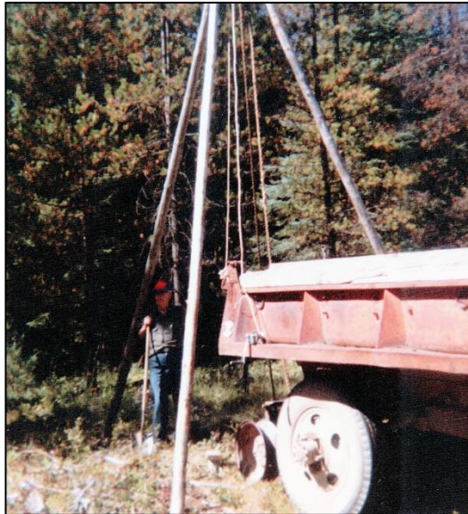
Ted Ross's well-drilling apparatus. Bob Olson helped Ross create roads and drill wells in the newly-platted Polebridge Townsite in the 1970s.
